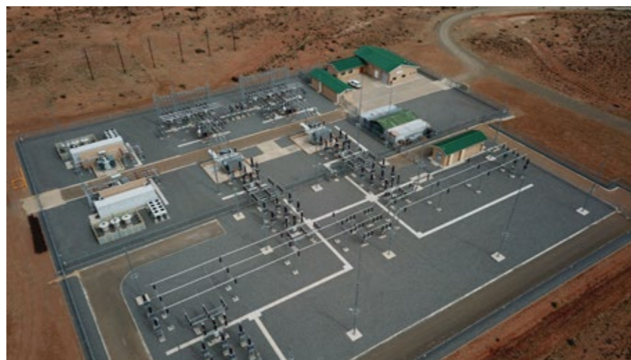
All electric transmission and transformation equipment are procured locally, increasing job opportunities for equipment manufactures and local community.
