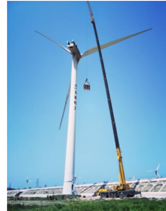
Longyuan Fujian Company Pingtan Wind Farm carried out the work of replacing the transformers of the unit to ensure the sound operation of the unit.
